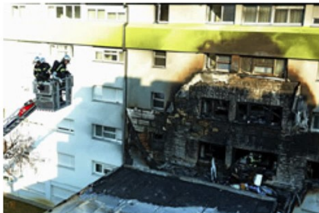
b) the façade after the fire was extinguished [11], [25]
